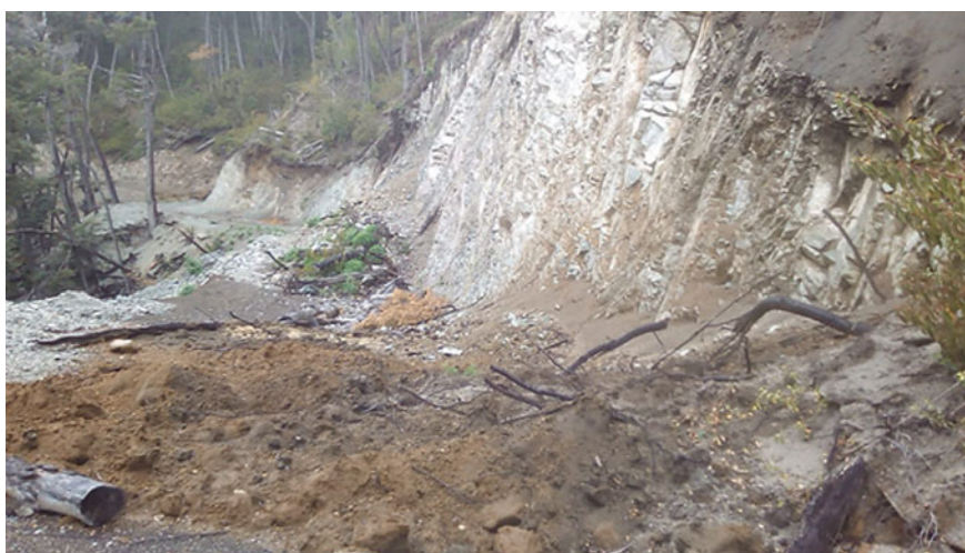
Fig. 5 Opening up a road in the area called Pichunco, Villa La Angostura, province of Neuquén, Argentina, 2019. Source Photograph taken by Gabriel Stecher
